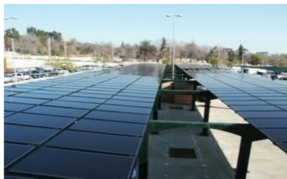
OMBRIERE PARKING CENTRE COMMERCIAL
